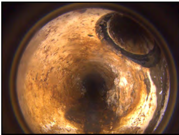
Figure 6: LS4_P121; Condition: 4; Deposits: Water Jet
