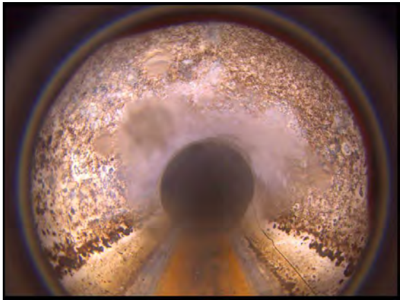
Figure 19: LS10_P065; Condition: 3; Spiral Crack
